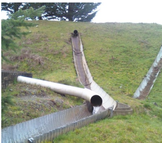
Outfall pipe. Source: courtesy of OGP members, 2014
