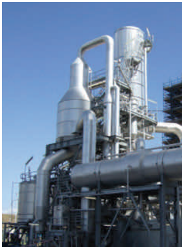
Advanced Treatment Facility : Crystallizer (Separation / Evaporation System)
