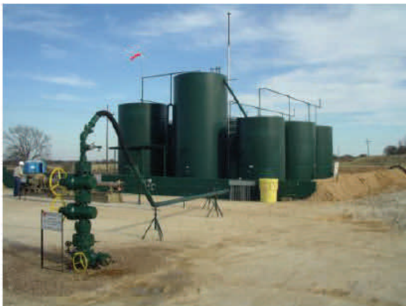
Injection well at Commercial Disposal Facility in Texas.
